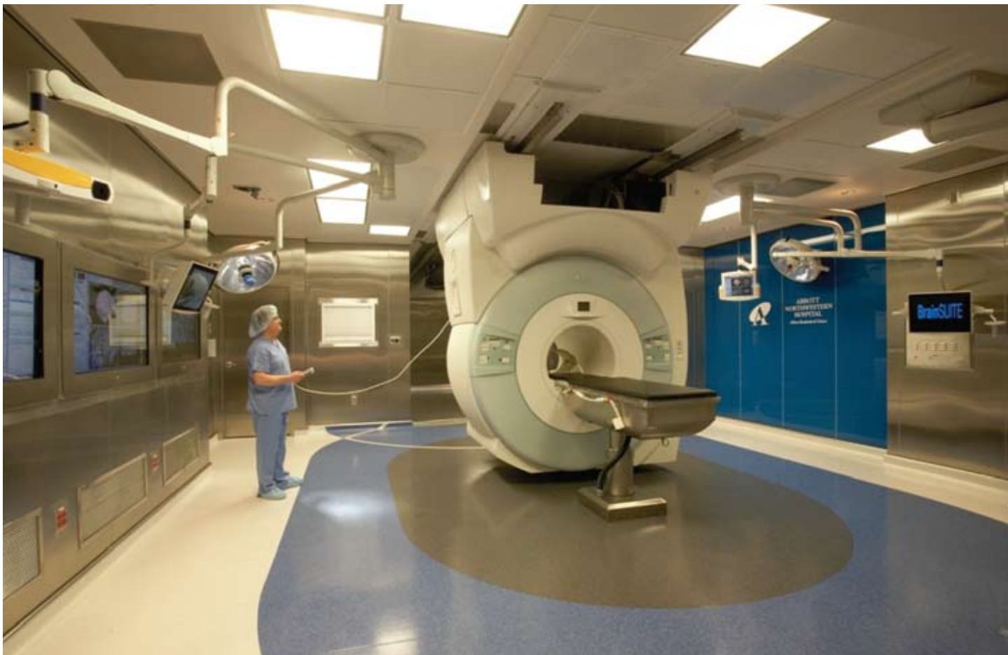
Abbott Northwestern's Intra-operative MRI was installed in 2007.
